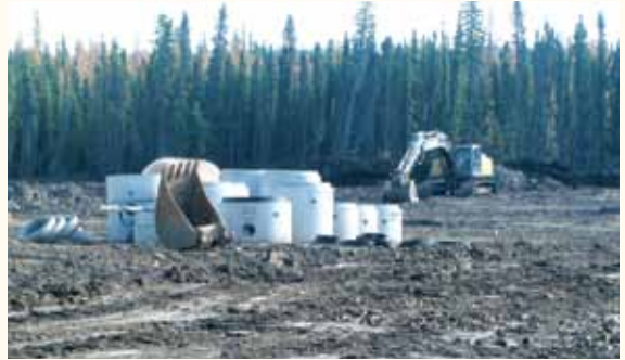
Construction began on the O'Chiese Truck Stop in 2009. Final completion is set for fall 2010.
